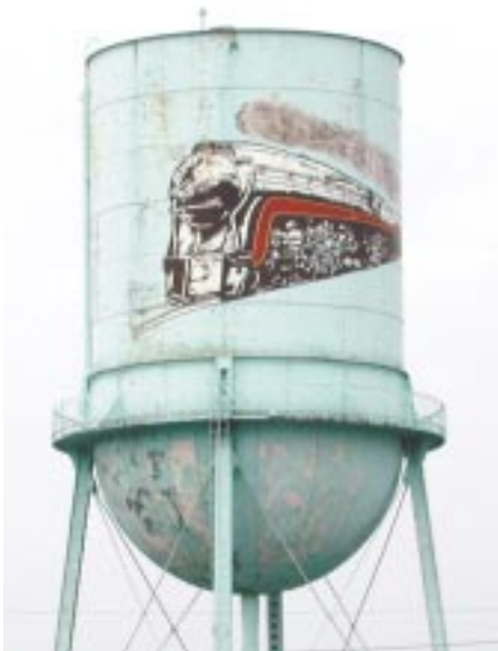
Crewe's distinctive water tower features a painting of a locomotive, reflecting the town's historic ties to the railroad.
